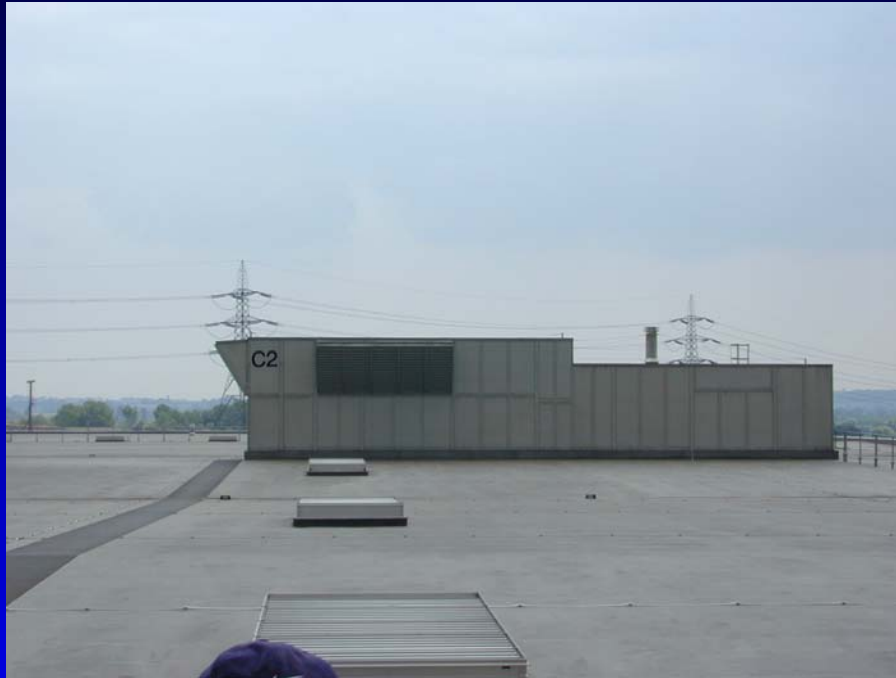
Roof-Top Air Handling Unit
