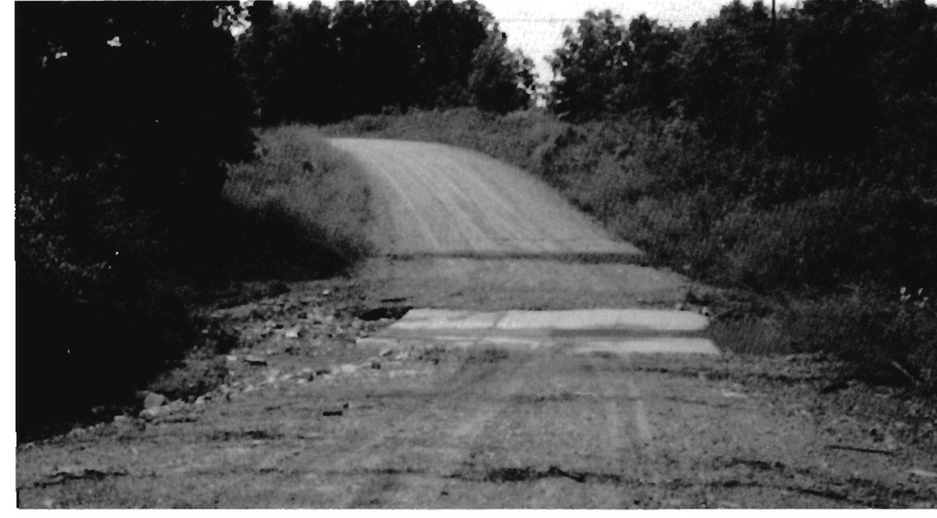
Concrete ford (Ford 22), located on Route 15, an all weather gravel road, at grid reference 787736. Concrete fords, eleven in all, are located throughout the reservation where erosion hazards are severe.
