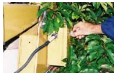
Picture 31 – Resetting emergency stop button
