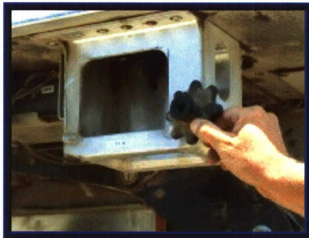
Photo 15. Loose Interlock Handle.
