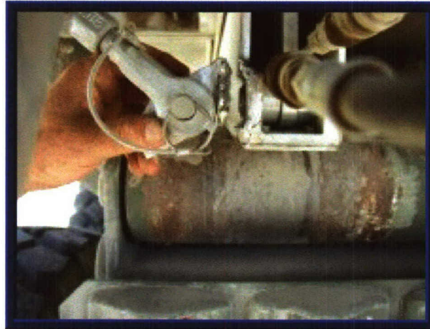
Photo 3. Broken Side Sway Bracket Weld.
