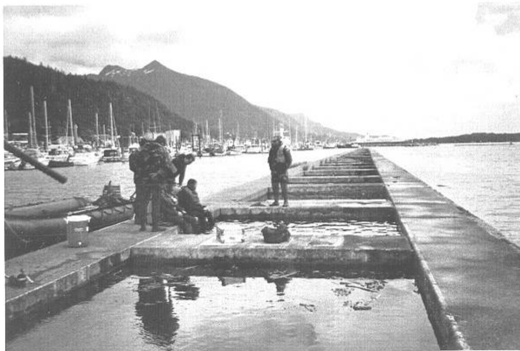
View of Misalignment Between Southern Most Modules
