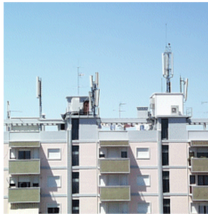
Figure 3 – BTS on the top of a building
