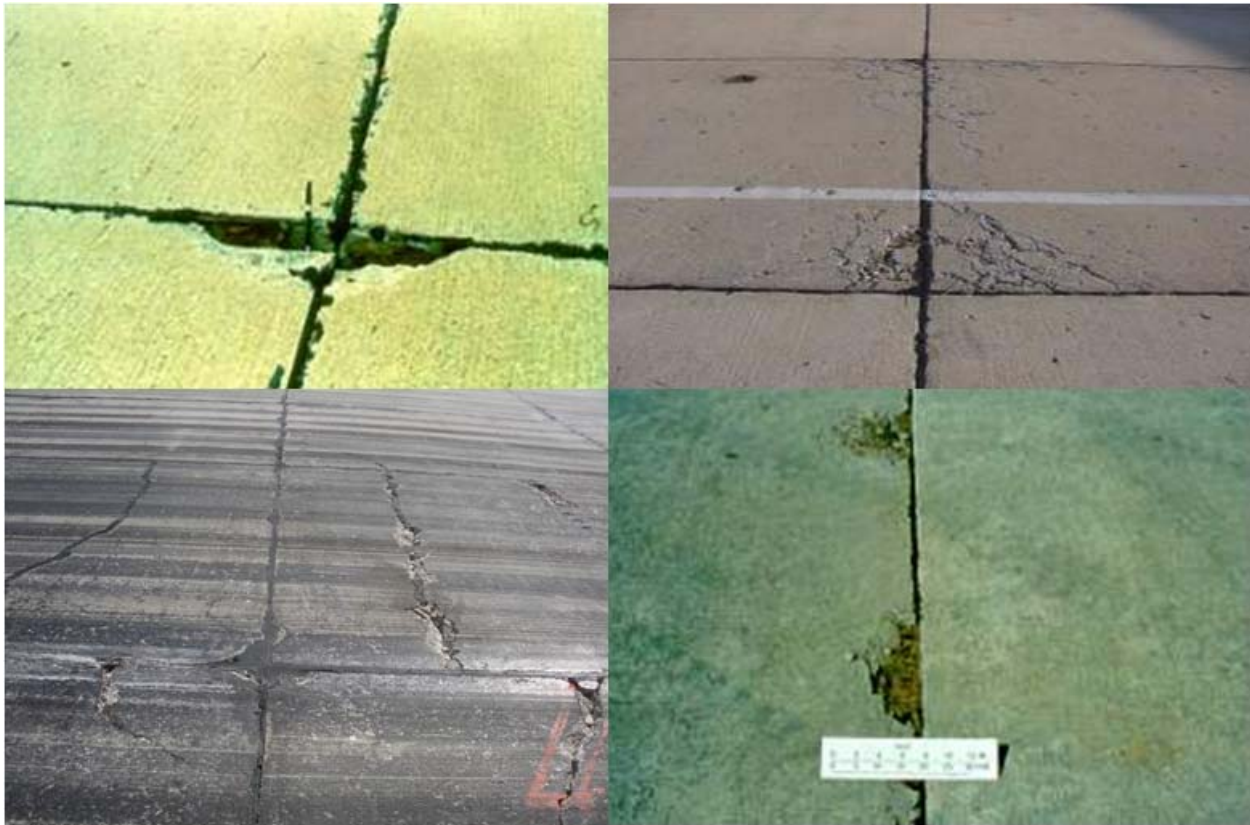
Figure 1. Concrete Pavement Spalls
