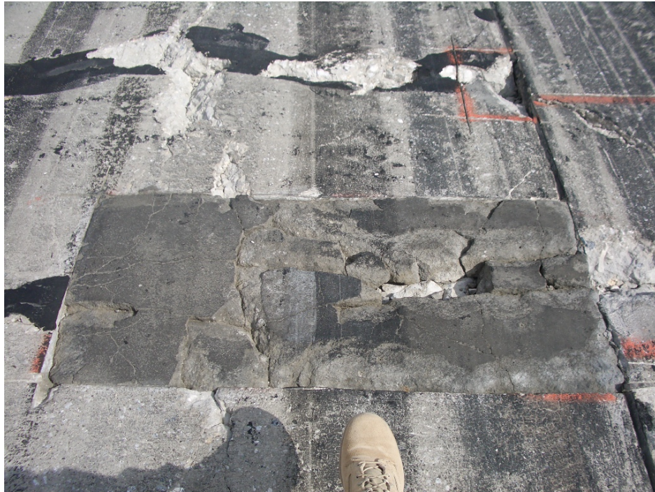
Figure 2. Example of a Failed Concrete Pavement Repair
