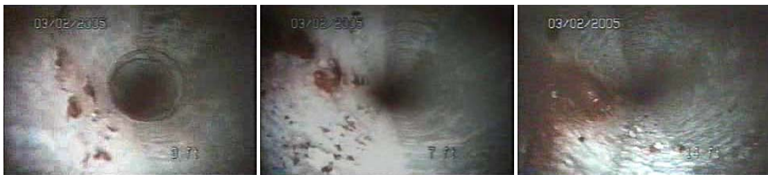
Figure 9. Pipe interior before treatment.
