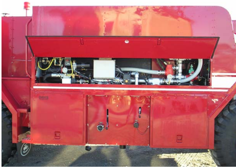
Figure 3.3.10: The UHP P-19's driver's side plumbing.
