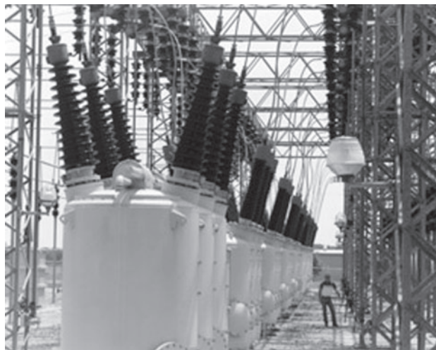
Source: Department of Energy. Power-generating plant switchyard.
