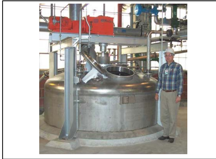
Figure 5-8. Secondary Containment "Dump" Tank
