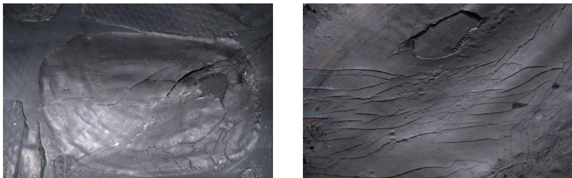
Figure 41: (L) The severely deteriorated repair patch located on the inner liner in a corner of the cell, and (R) typical cracking found on the repair patch
