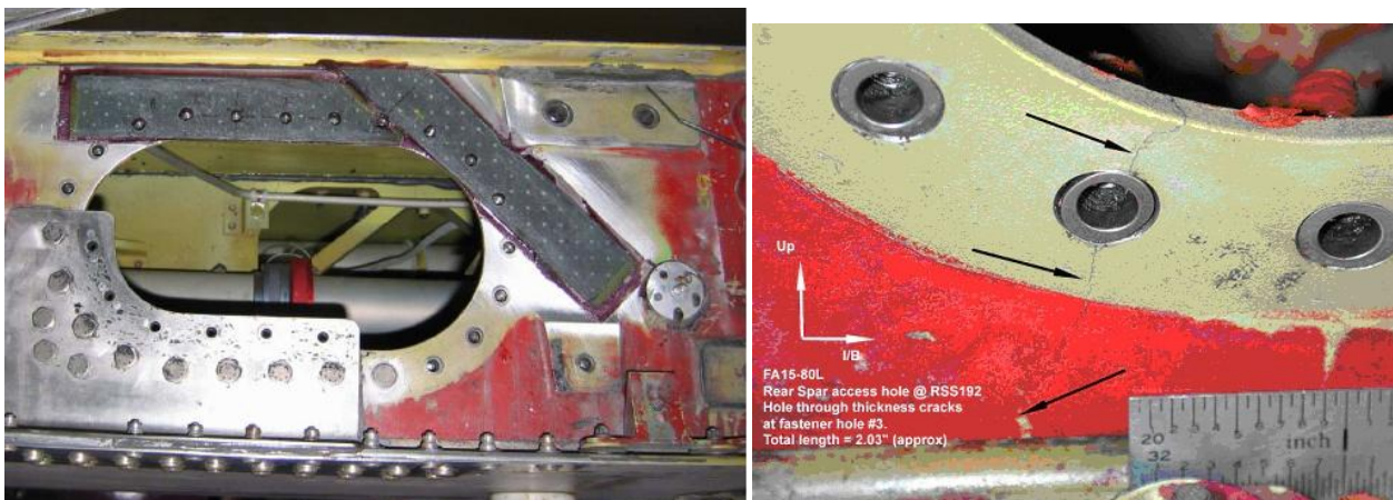
Figure 6: Boron Doublers Fitted to the DI 73 Cut Out to Inhibit Crack Growth
