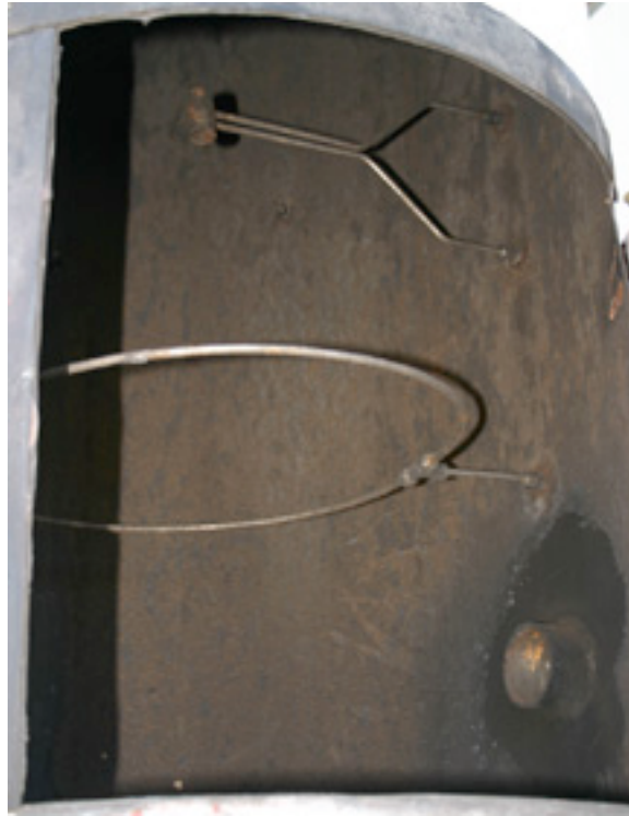
Figure 5. Interior of Calorimeter Exhaust Duct
