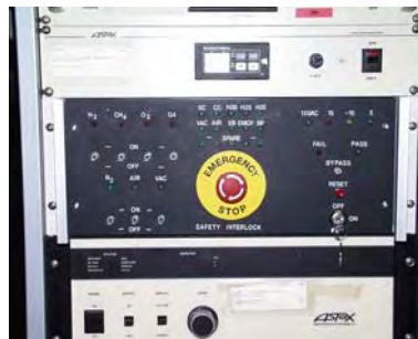
Safety Interlock System
