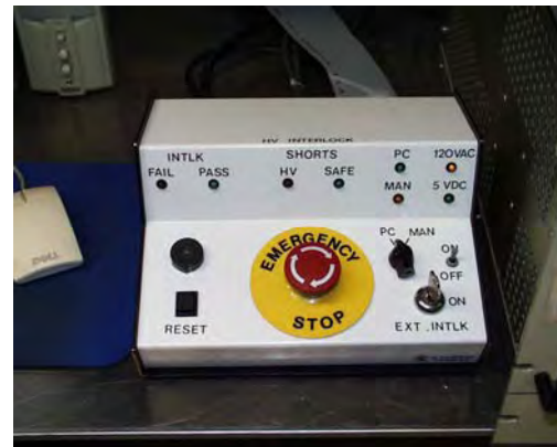
Safety Interlock System
