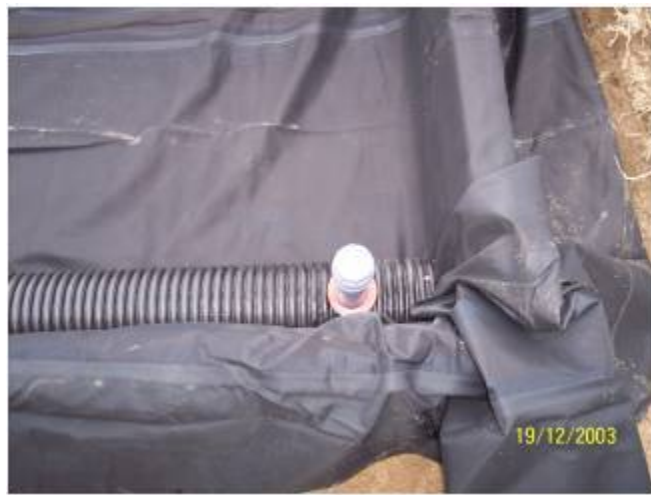
Figure 19. View Port of Water Collection Reservoir.
