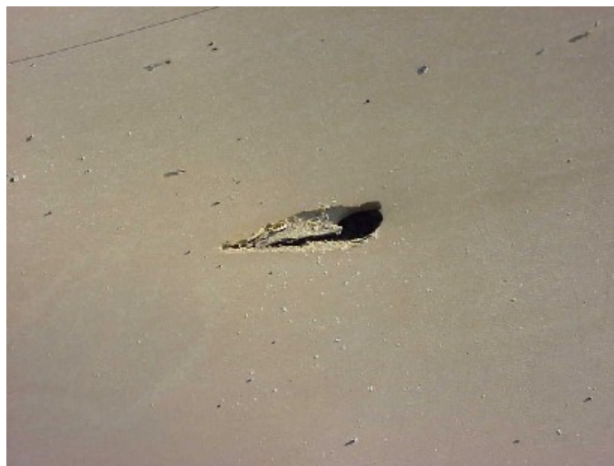
Figure 34. Damage on Left Side of Range 5.
