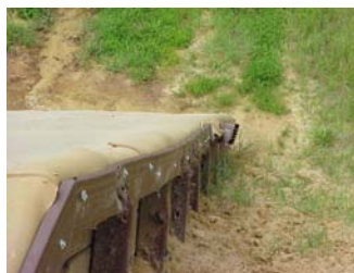
Figure 44. Loose Plank on Left Side.
