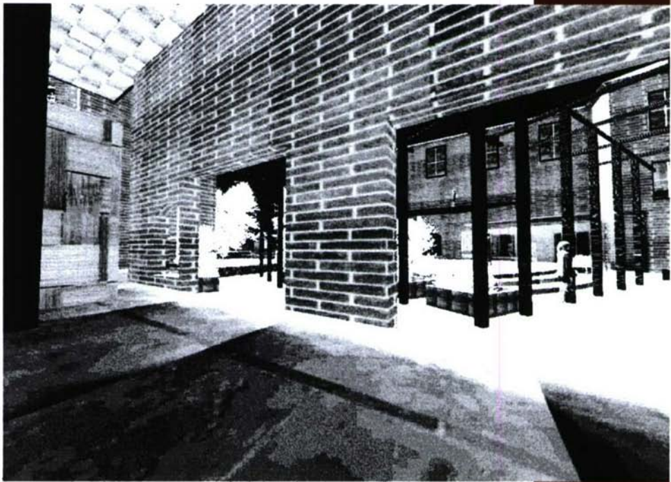
Interior of Kitchen Classroom showing openings where large garage overhead doors will be installed to open directly to herb gardens on terrace
