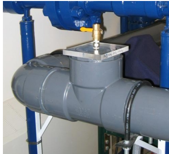
(a) Pressure Relief Plate and Vent Valve
