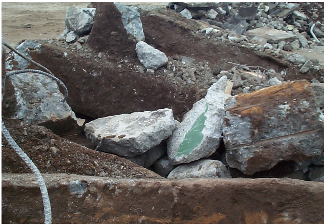
Figure 13. LBP covered concrete in mixed debris pile.
