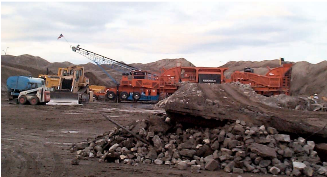
Figure 1. Overview of crusher plant.
