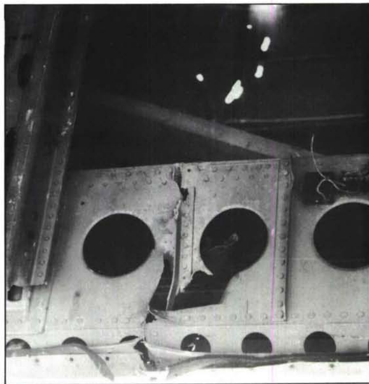
FIG.22f. STARBOARD SIDE. NOTE:- BUTTING OF SEVERED MEMBERS
