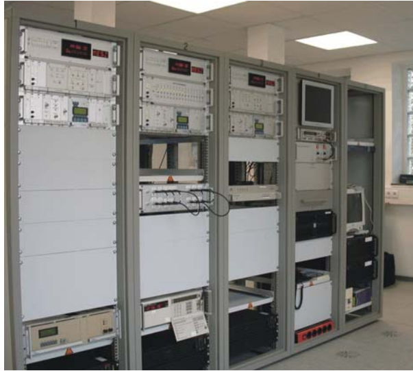
Figure 1. New electronic control during construction. As a detail, one can see in racks 1 to 3 the three signal generators and temporarily only two atomic frequency standards.
