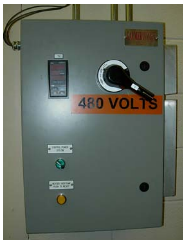
Fig. 11. Gaumer electric heater circuit breaker
