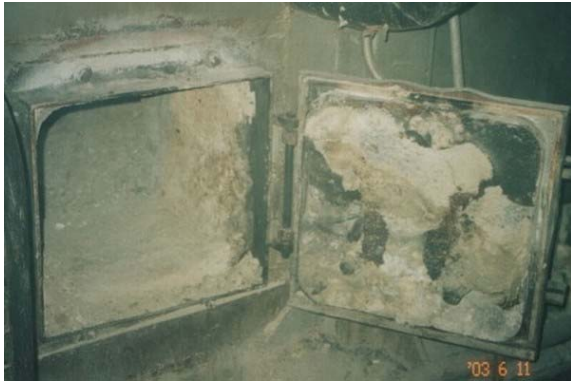
Dr. 1. Refractory concrete BRAB30И15 boilers hatch without protective covering after 2 months of operation, june 2003.
