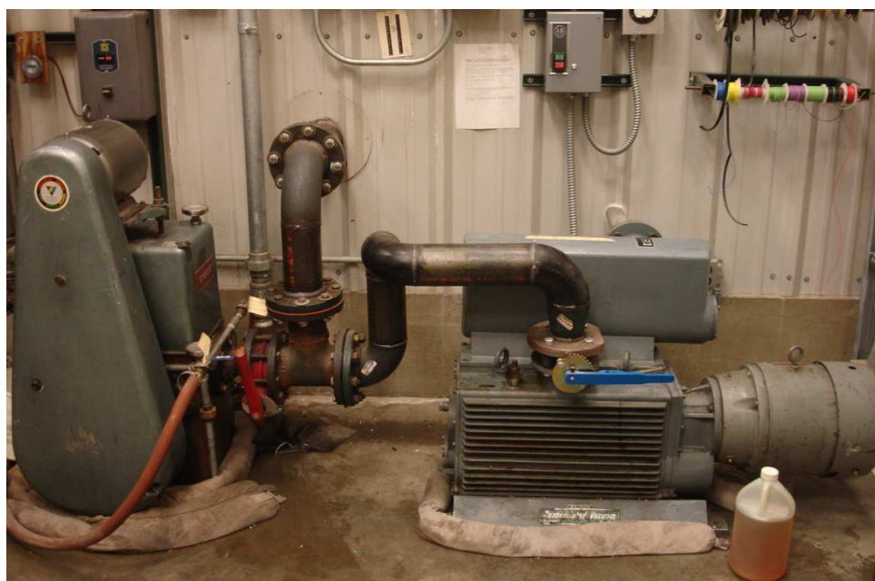
Figure B.7: PQFLT facility, vacuum pumps
