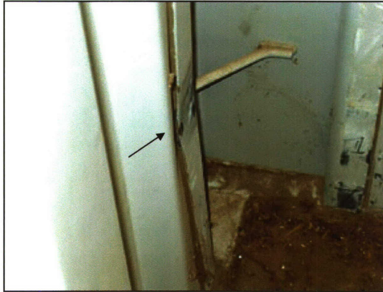
Photo 7. Damaged Container Corner Post
