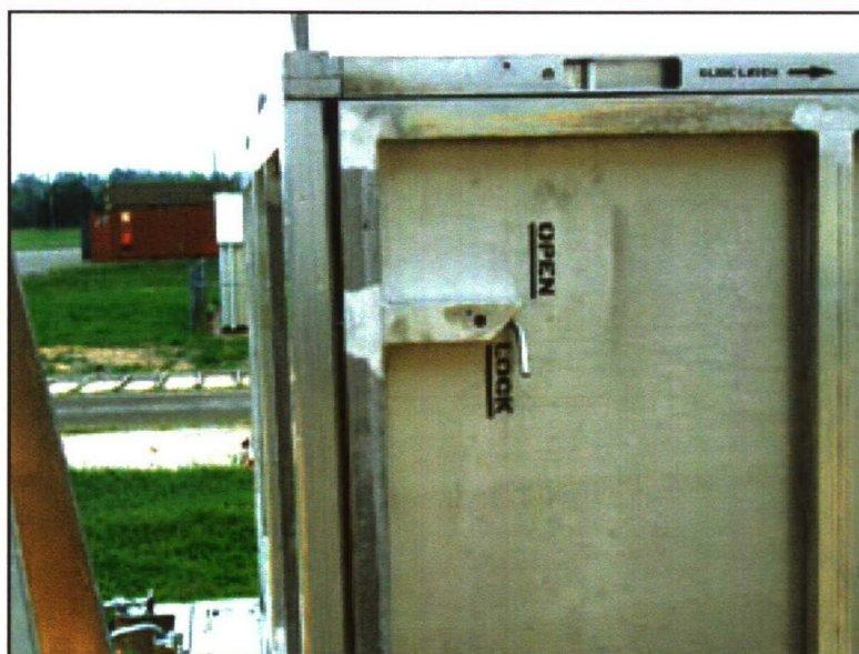
Photo 16. Partially Disengaged JMIC Door Lock
