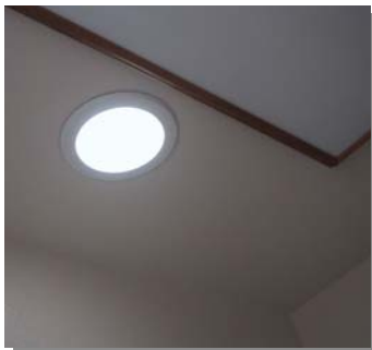
Figure 5. Solar tube skylights.
