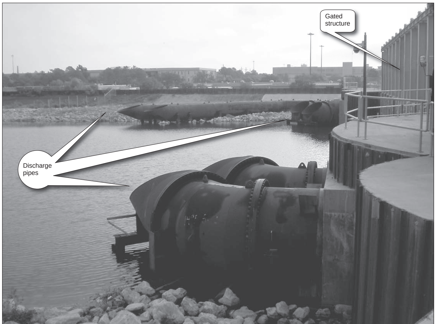
Figure 7: Discharge Pipes at the London Avenue Canal
