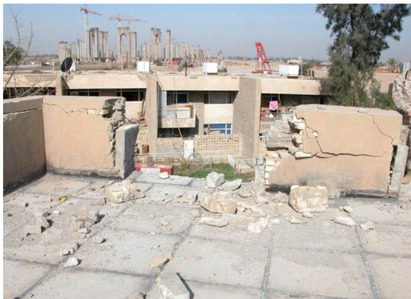
Figure 2 – Roof of Bombed Baghdad Recruiting Station
