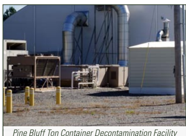
Pine Bluff Ton Container Decontamination Facility
