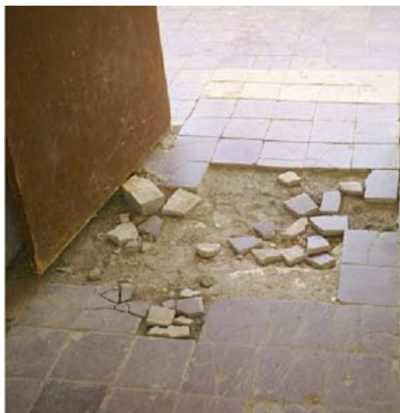
Broken tiles in school classroom
