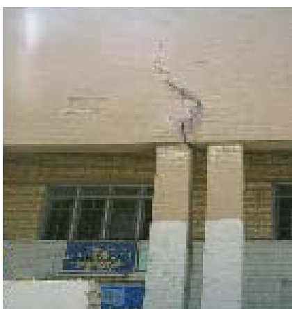
Cracks in school's outer wall
