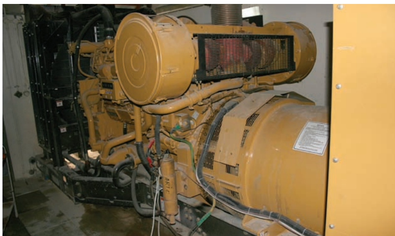
New generator used as a back up.
