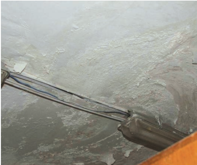
Water damage to the ceiling.
