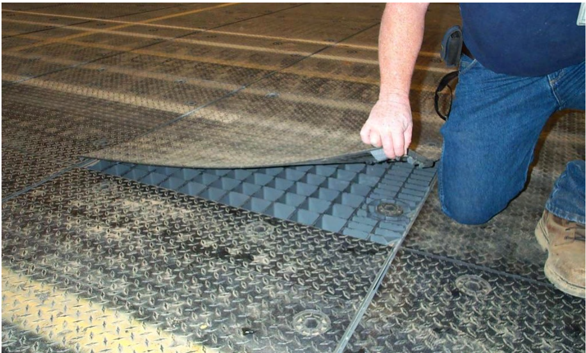
Photo 33. Delamination Failure of the BRAVO® Mat While Installed on SM Test Section
