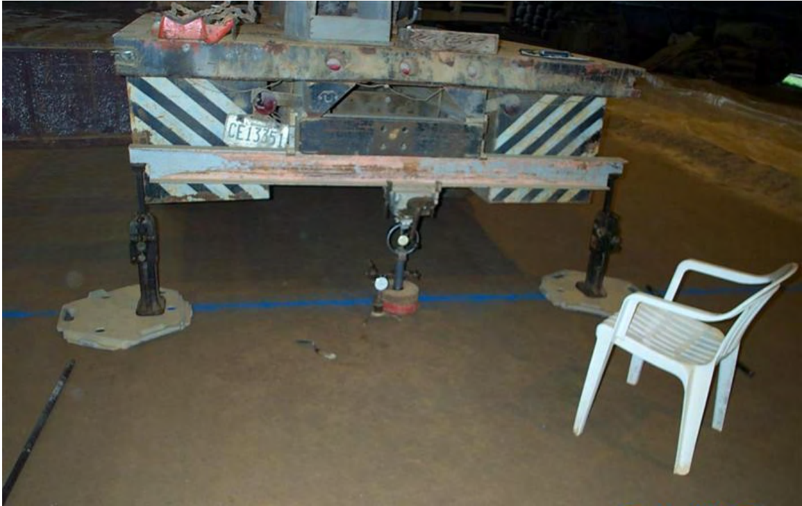
Photo 16. Typical Field CBR Setup on the Finished SM Blend Test Section Surface
