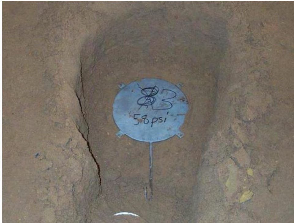
Photo 21. Geokon Model 3500 Pressure Cell Being Installed in the Medium Strength Test Section
