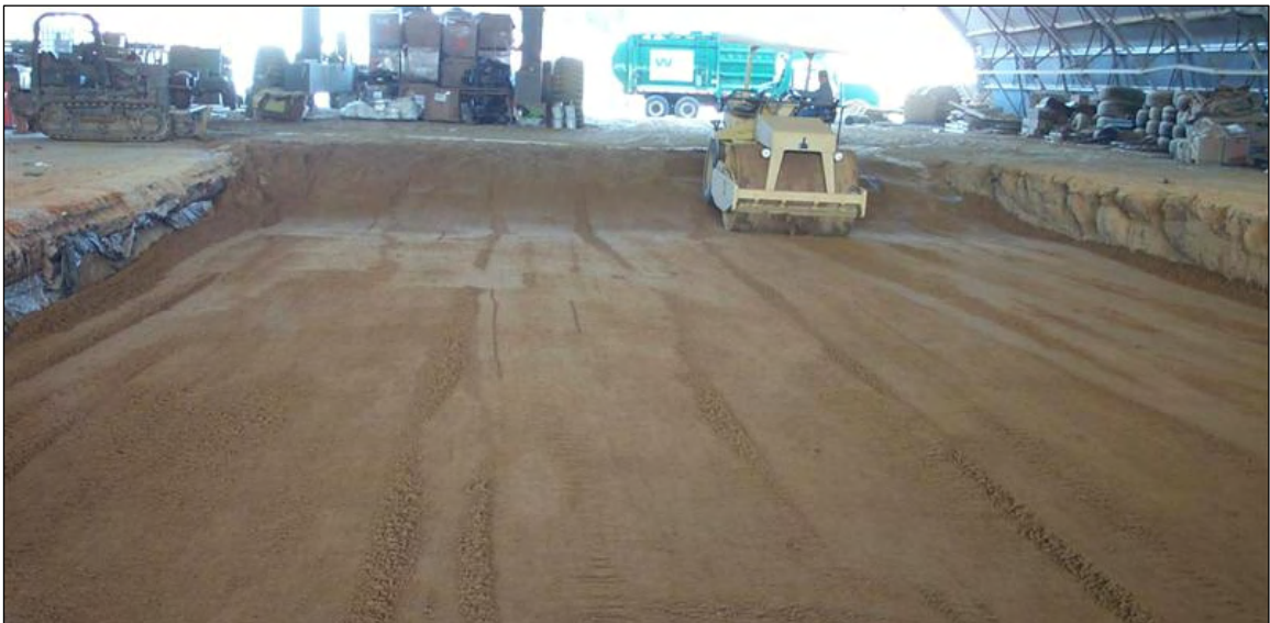
Photo 15. Installation of SM Blend in Test Section – Finish Compaction with the Vibratory Steel-Wheel Roller – Installation 50 percent Complete in this photo.
