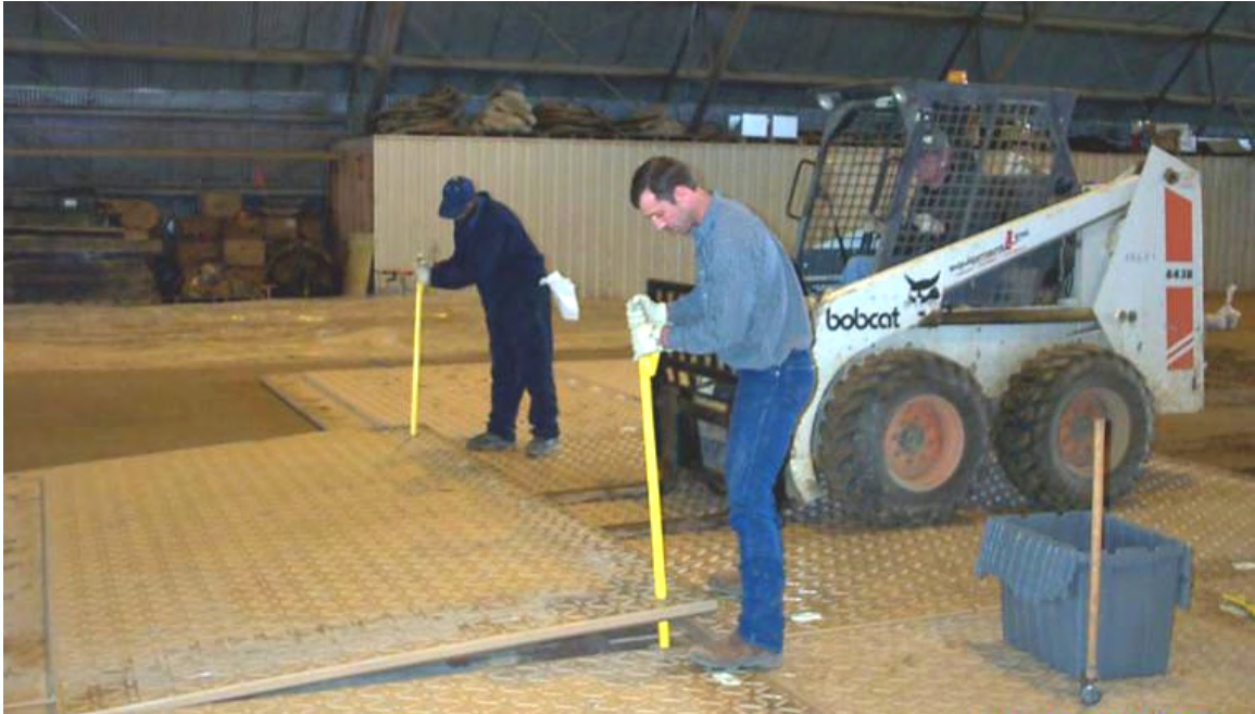
Photo 8. Dura-Base® Mat Being Assembled on Medium-Strength Subgrade Test Section (Note: the Yellow Rods are Used to Align the Mat Holes for Pin Connection)
