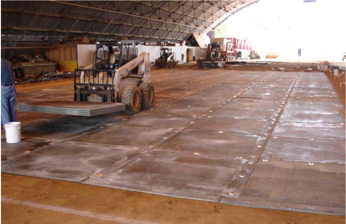
Photo 13. ACE-Mat™ on the Medium-Strength Subgrade Test Section (Note the underlap and overlap pattern of the mat edges)
