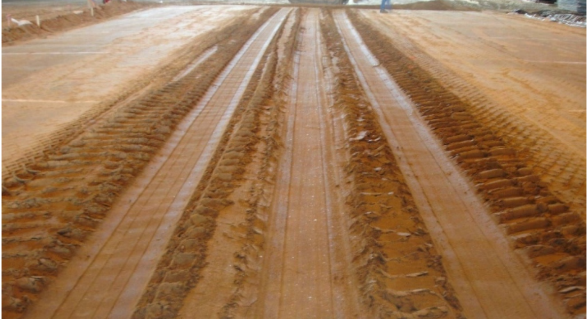
Photo 27. Silty Sand Control Test Section After Rutting Failure
