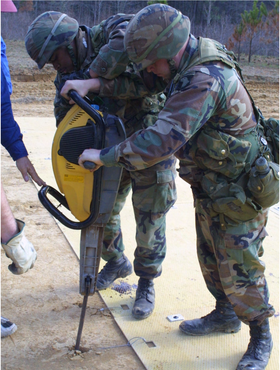
Photo 12. Gasoline-Powered Hammer-Drill Being Used to Install Duckbill Anchor— These Soldiers were involved in an Exercise Separate of JRAC
