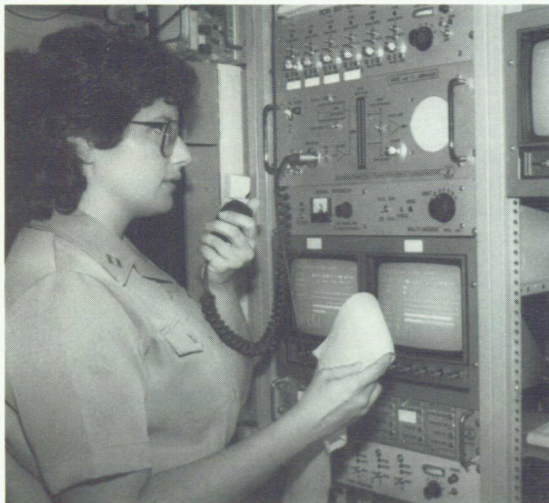
Shore electronics instrumentation yields data from cable fields during Atlantic Ocean tests.
