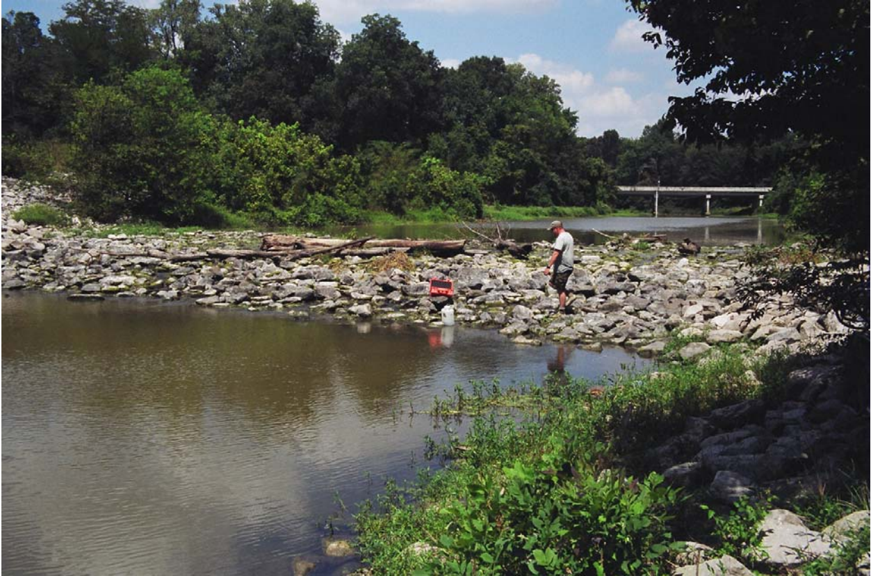
Figure 6. Low-crest rock weirs with long, tapering slopes provide excellent habitat conditions for delta stream fishes at a relatively low cost.
