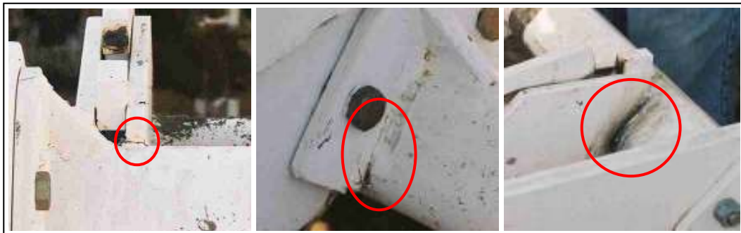
Figure 23: Cracks Found on the MCC
