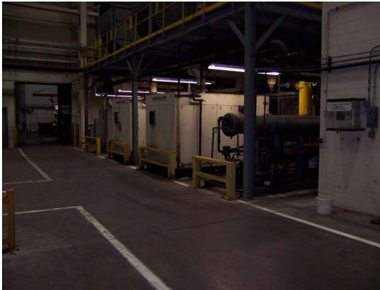
Figure 27. Three Air Compressors in Building 222.
