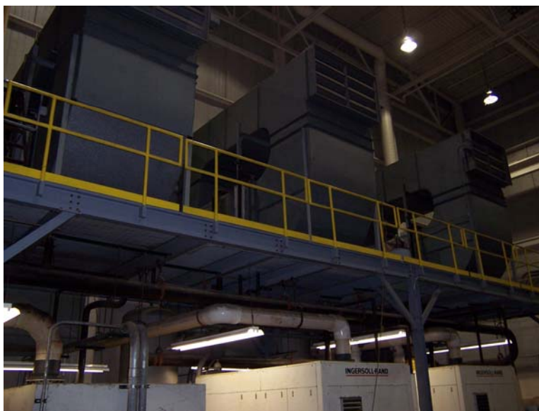
Figure 28. Air Compressors with air-cooled heat exchangers above.
