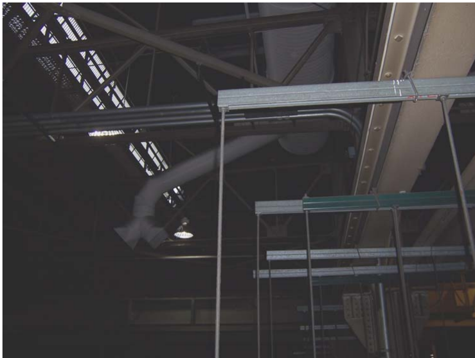
Figure 15. High level diffusers in Heat Treat.
