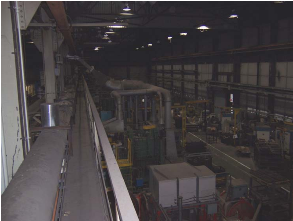
Figure 16. Heat treat area showing exhaust systems
