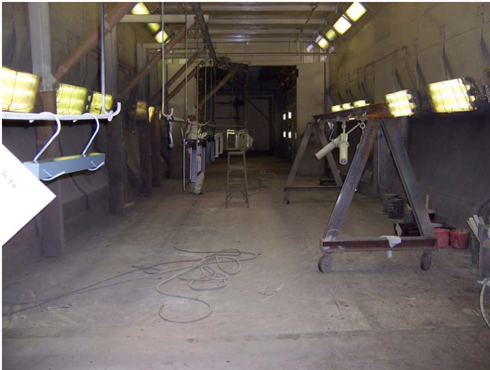
Figure 11. Paint Booth # 2 in B-208.
