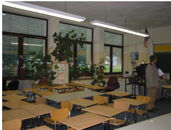
Figure 37. Original suspended luminaire lighting system.
