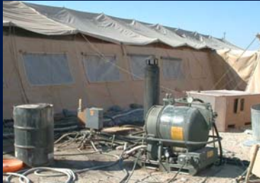
Water heater fueled by JP-8
