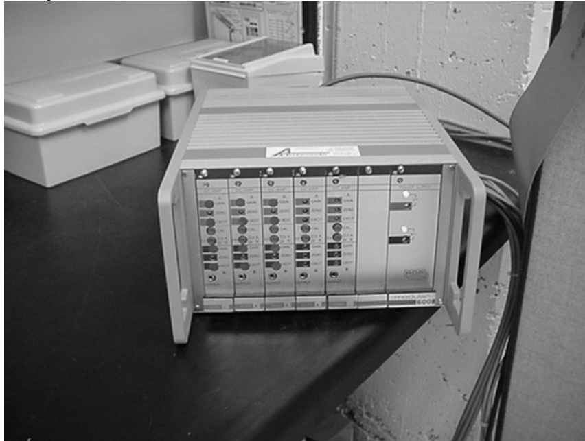
Figure 7. RDP Group Modular 600 Amplifier
