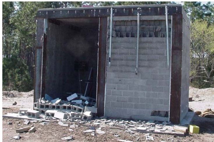
Fig. 3.1-3: Wall damage after the test
