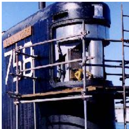
Fig. 2. HF active sonar array mounted in the sail of the USS Asheville, a 688i Los Angeles Class submarine (From N77, 2002).
