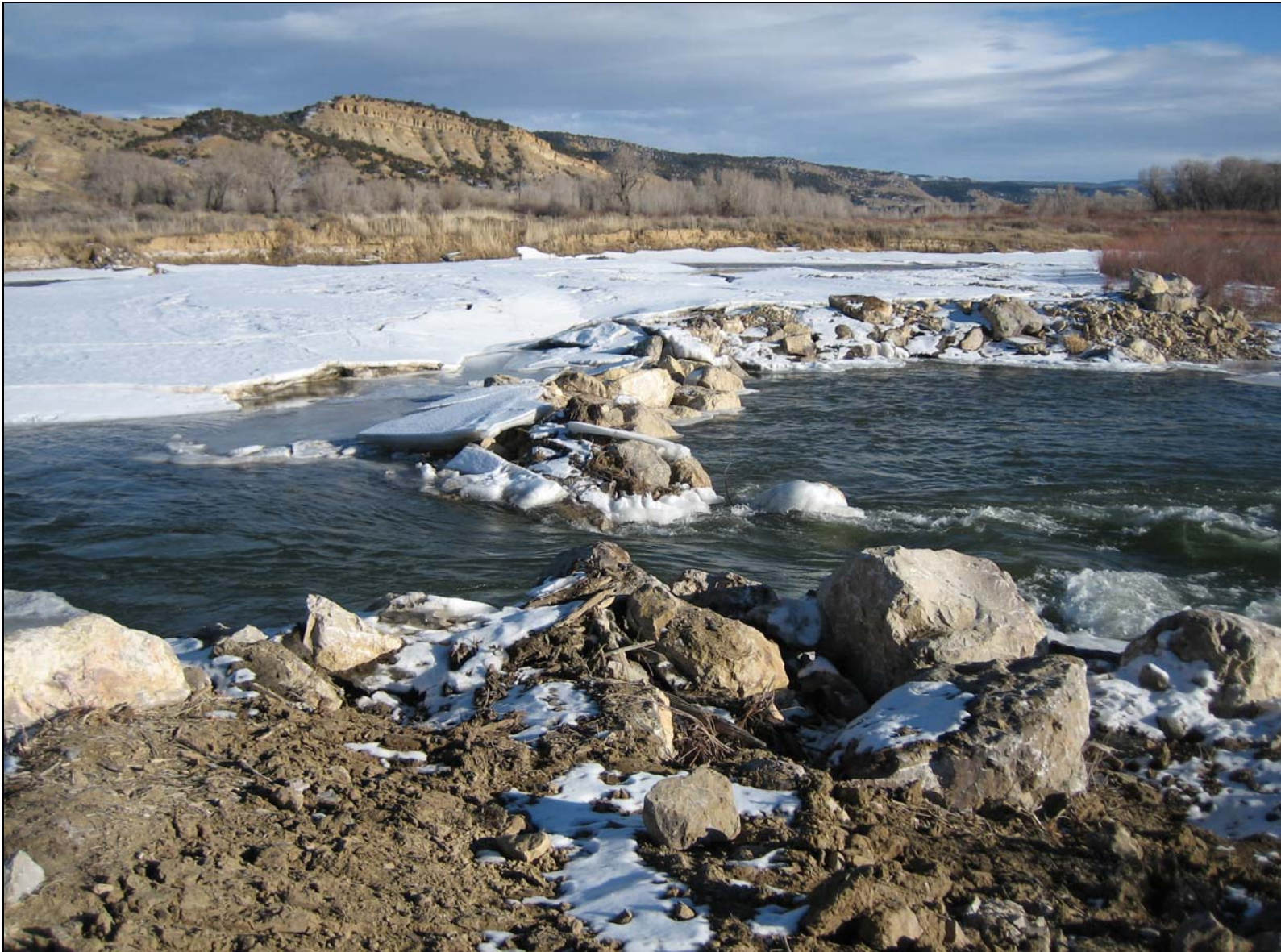
Figure 14. Breached CDOW rock weir, 17 January 2006.
