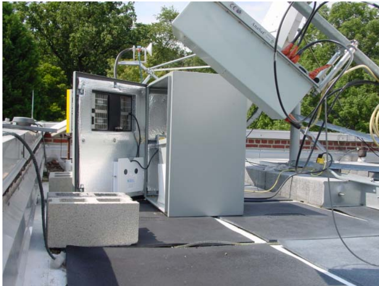
Figure 8. Thermoelectric all-weather chamber for TWSTT electronics.
