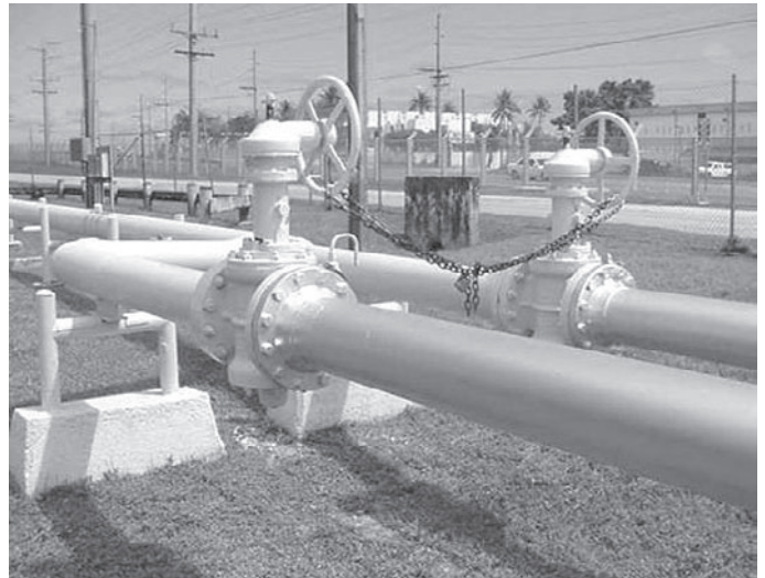
Fuel transfer pipeline.
