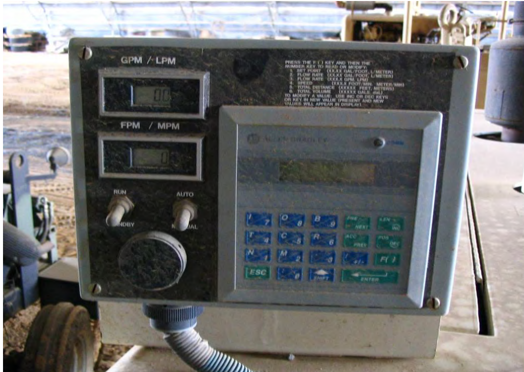
Figure 31. Control box for the liquid proportioning system.
