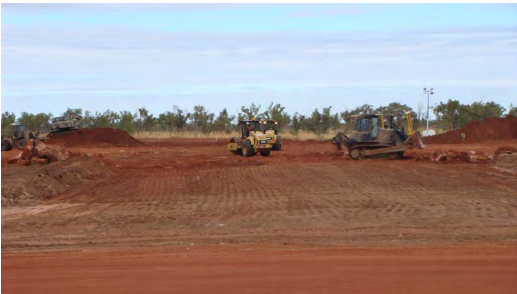
Figure 73. Box out of Taxiway and Apron Bravo after first rain event (23 June).
