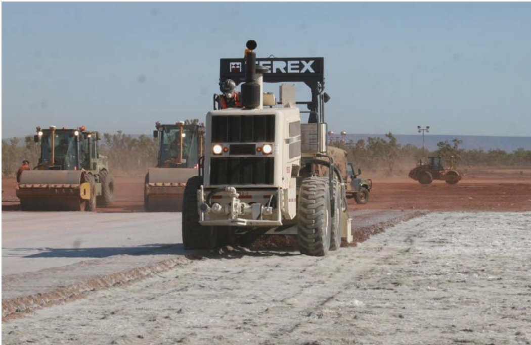
Figure 82. Terex 350RS mixing soil with fiber and cement on Apron Bravo, 27 June 2007.
