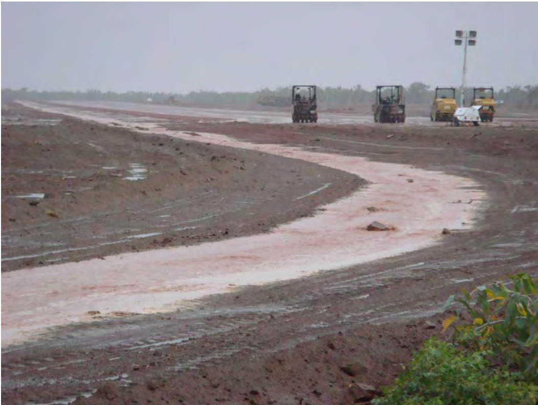
Figure 74. Drain from Taxiway Alpha to edge drain on primary runway.
