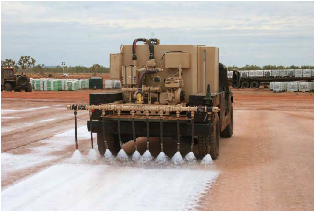
Figure 83. Application of polymer emulsion surface cap on heliport using a HUMVEE sprayer.
