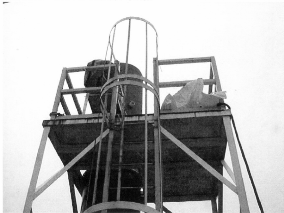
FIGURE 2. LINE 2 EXHAUST STACK
