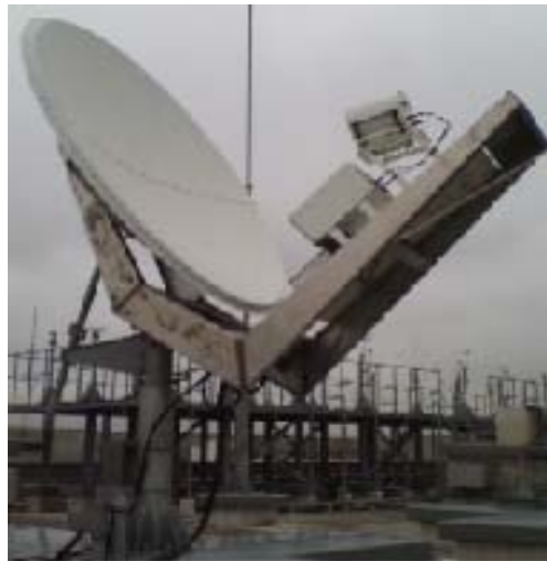
Figure 4. The antenna and the outdoor unit of a fixed TCE Earth station.
