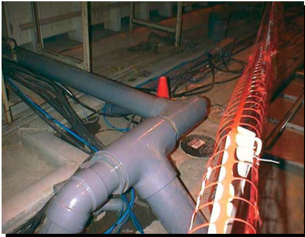
Figure 2. Main VR Piping Inside Building 181
