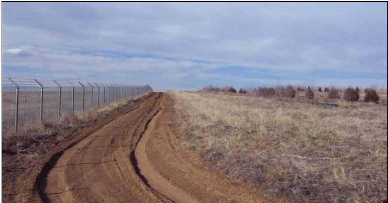
Figure 1-2. Ungraveled Portion of Perimeter Road After a Rainstorm
