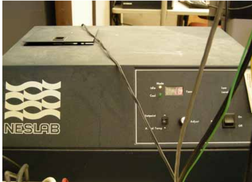
Figure 4.2: NESLAB model HX-75 chiller.
