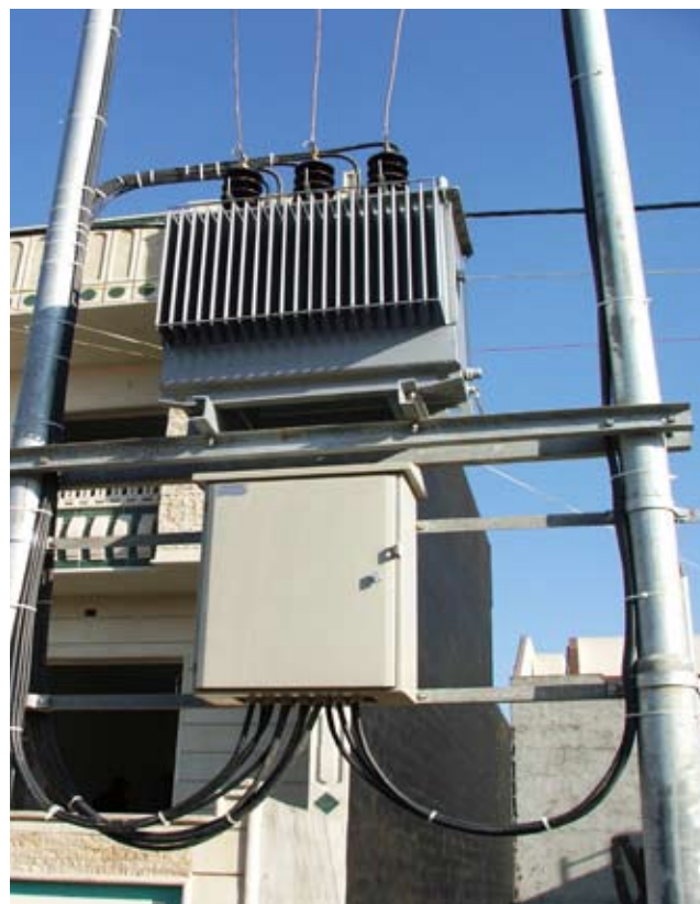
Transformer and low voltage electrical distribution panel
