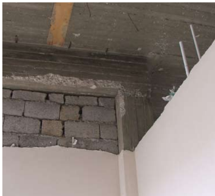
Segregation of load-bearing reinforced concrete ceiling beam
